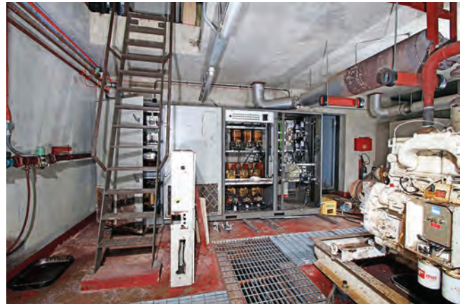
The generator room on the lower floor; the cabinets at the rear appear to be wrecked. The machinery entrance blast door is seen on the right
